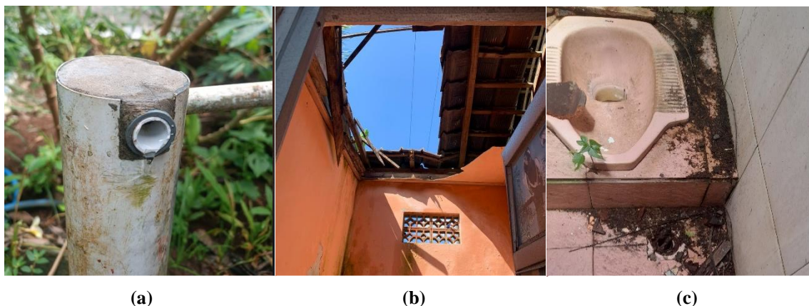
Figure 1. Inadequate WASH and MHM Facilities. (a) Broken pipe. (b) Severely damaged student toilet. (c) Dirty toilet.
